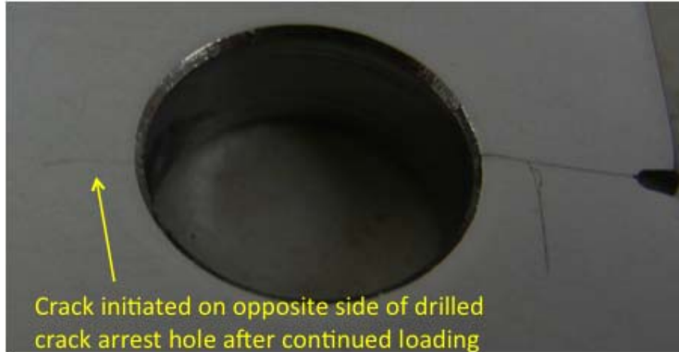
Figure 10. New Crack That Initiated After Being Drilled with a Crack Arrest Hole
