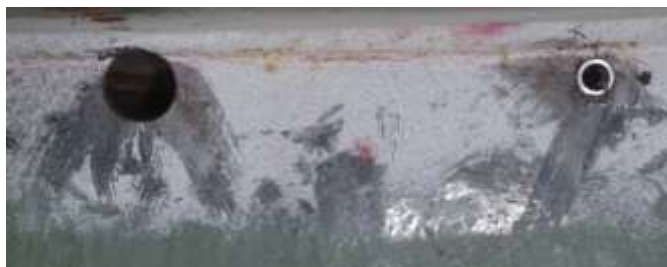
Figure 16. Typical Crack Arrest Hole at One End of Crack and StopCrackEX on the Other
