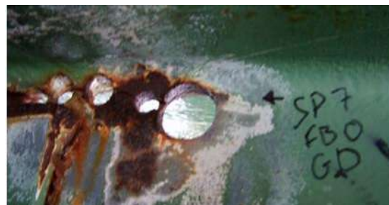
Figure 1. Photo of Multiple Attempts to Arrest a Crack
