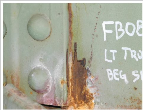
Before Repair: Location of Crack
