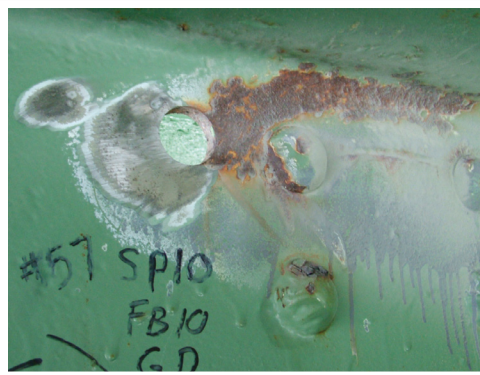
Typical Crack Arrest Hole
